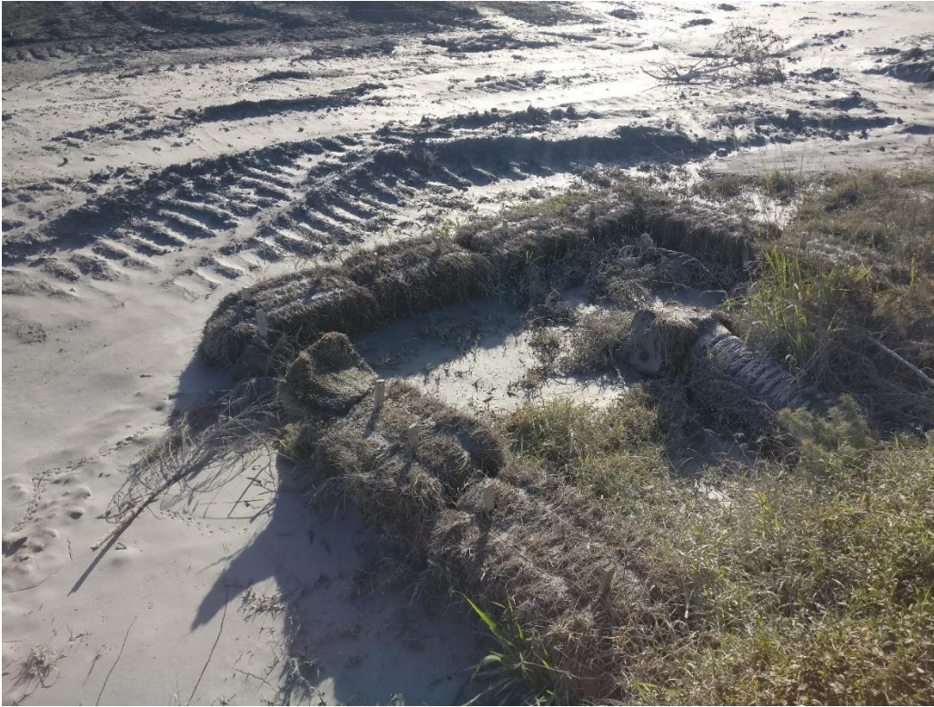
Figure 7. Damaged and Displaced Hay Bales in Cell 1
