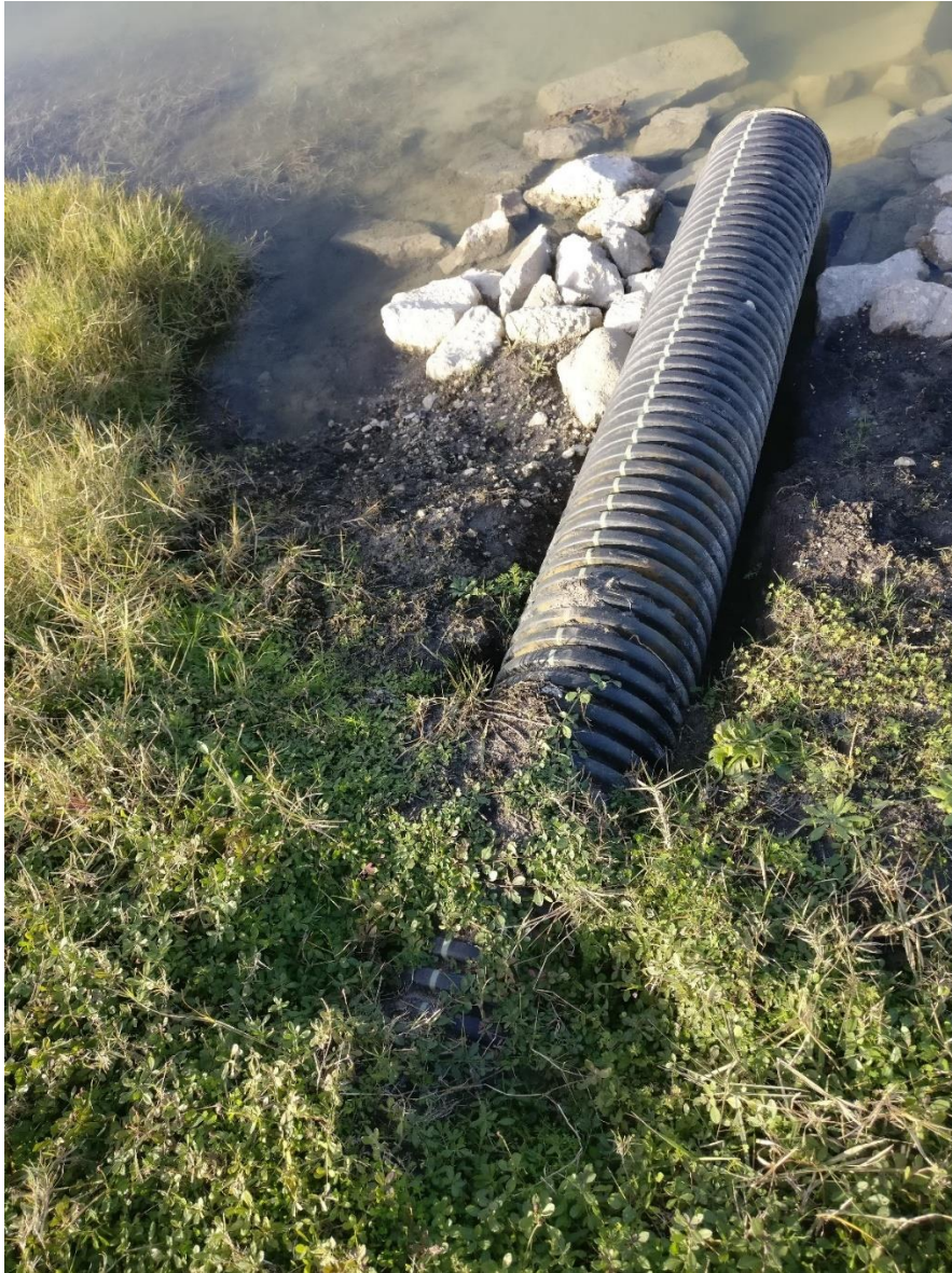
Figure 8. Erosion around Downcomer Outlets
